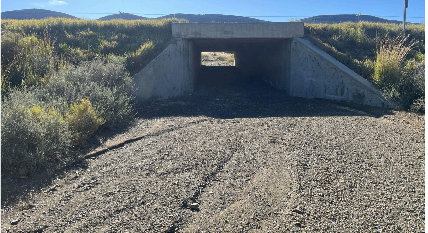
Figure 4.16: One of the current culverts. The streambeds all consisted of fine sand with rocks that were easily carried downstream
